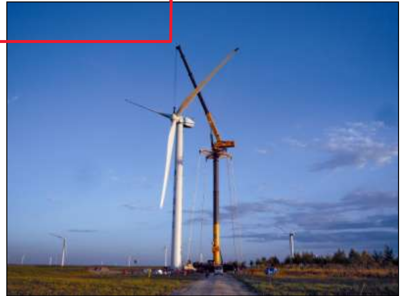
GTK 1100 at wind farm in China.
